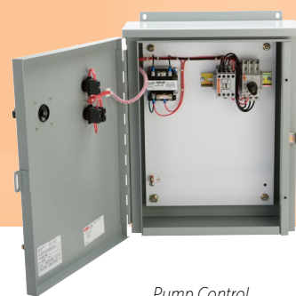
Pump Control Panel
